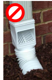
Uncovered filter not permitted
